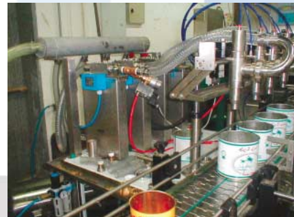
Coriolis in action at an olive oil canning factory
