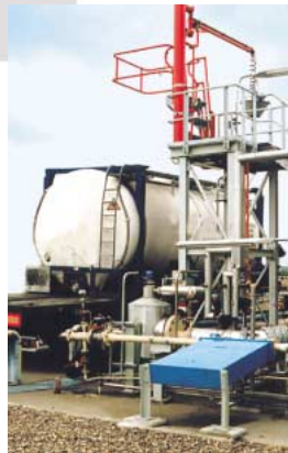
Highly accurate truck filling station with RHM 60 FNT for custody transfer
